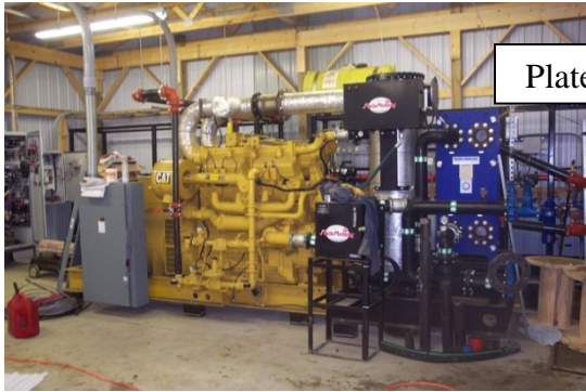
Partially Installed Engine Skid
