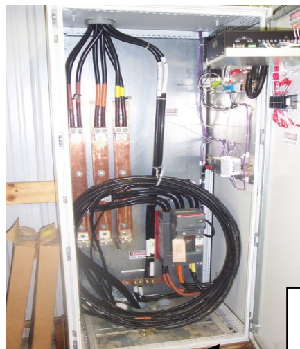
Engine Control Panel
