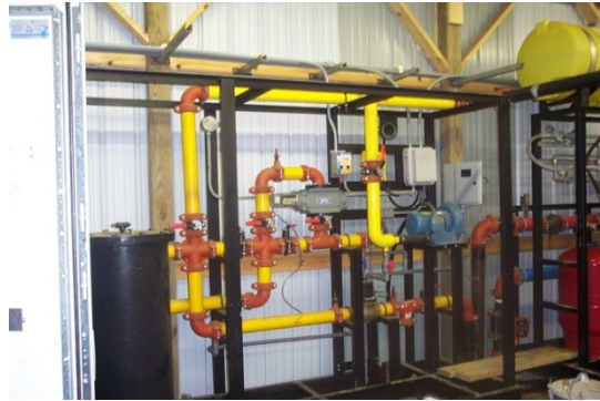
Biogas Conditioning Skid
