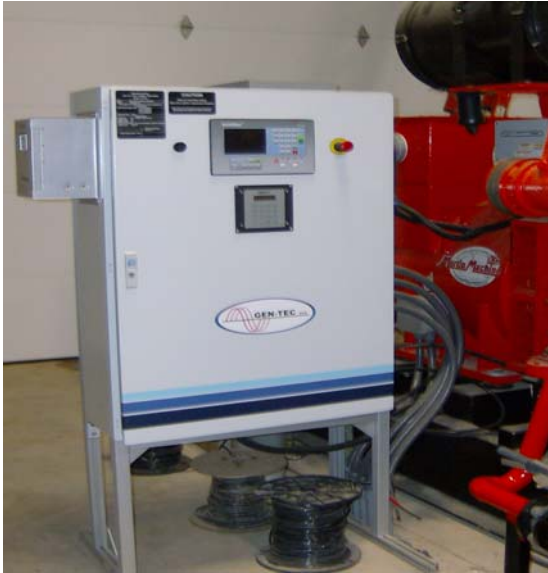
Gentec engine control panel.
