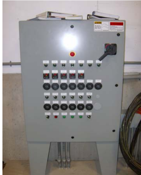
Digester control panel.
