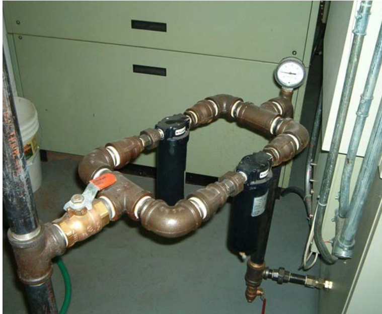
Figure A1 Dual 1/2 Inch Natural Gas Filter Assembly
