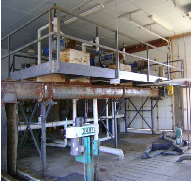
Separators and conveyor system
