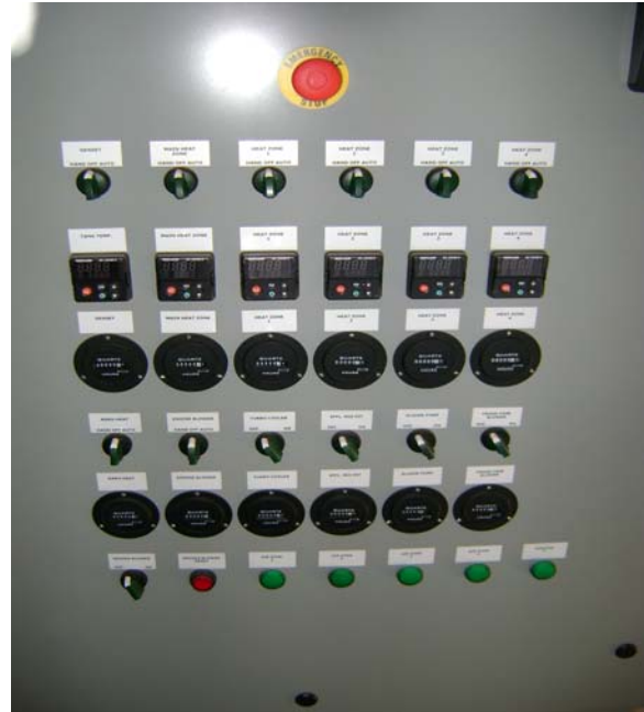
Digester Control Panel (from GHD)
