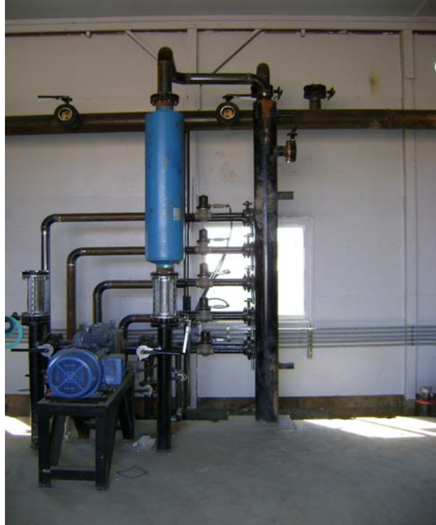
Biogas blower (25 HP) and piping for digester mixing
