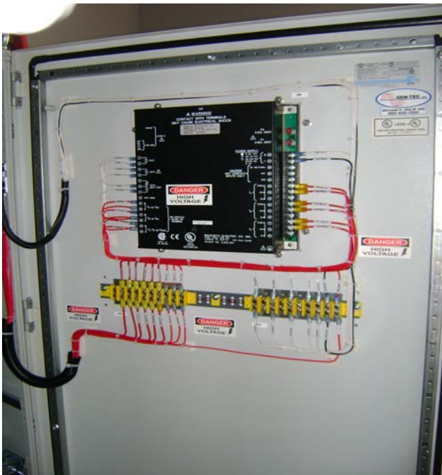
Beckwith Protective Relay (from back of door)
