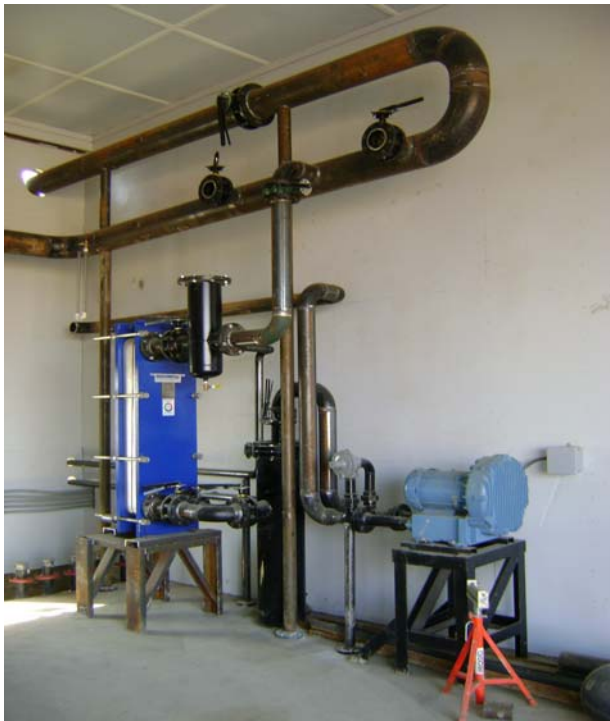
Biogas cooling heat exchanger; 7.5 HP Blower, Piping to Flare
