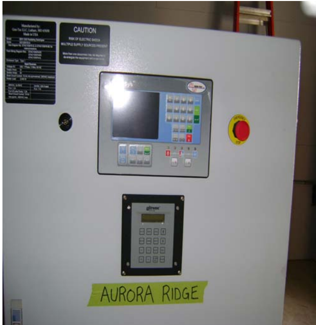
GenCon II Panel w/ Power Meter
