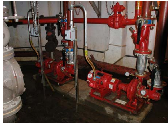
Hot Water Heat Pumps in the Digester Control House Basement
