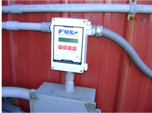
Fox FT2 Flow Meter – “Passive” Flare (FGF)
