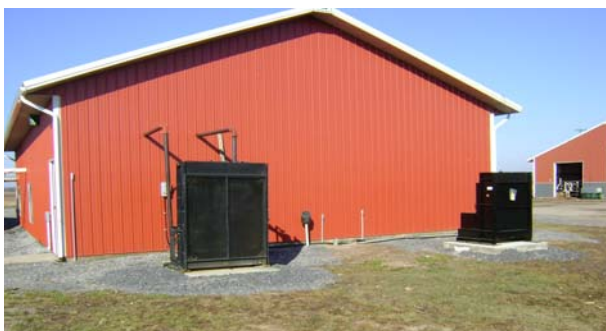
Engine Radiators Next to Pole Barn
