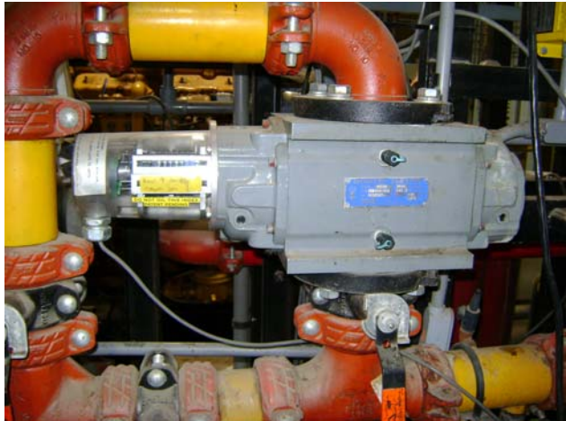
Roots Gas Meter – Existing ENGINE (FGE1) (now removed)
