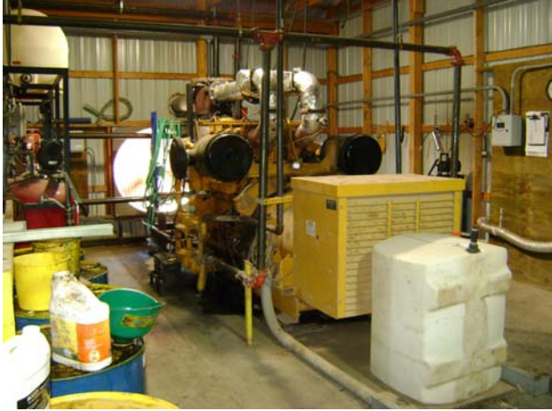
Original (existing) engine - Cat G379
