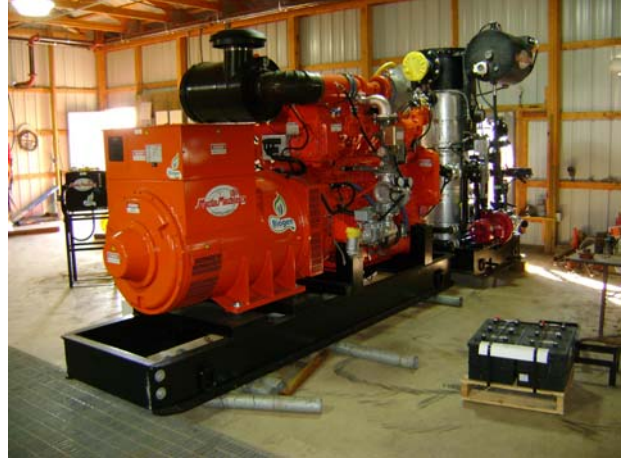
New engine - Guascor SFGLD 180
