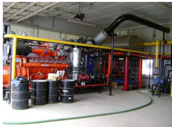
Installed Engine-Generator Set
