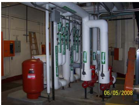
Installed View of Heat Exchangers
