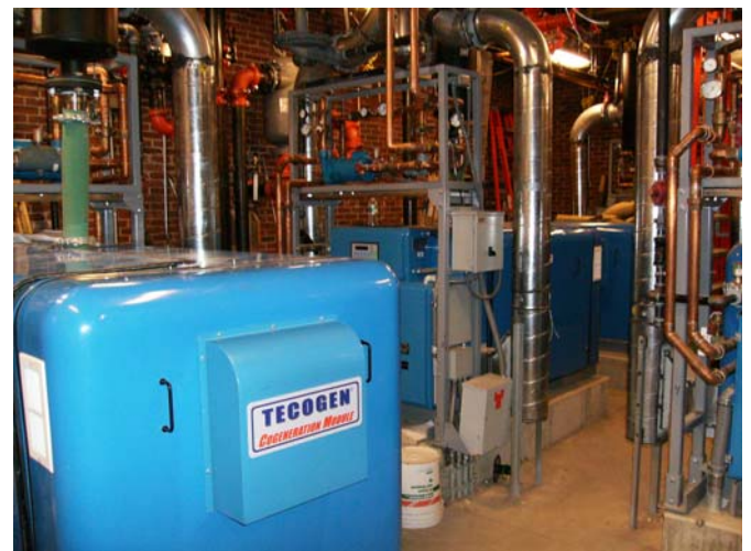
Installed 75kW Engine Generating Sets
