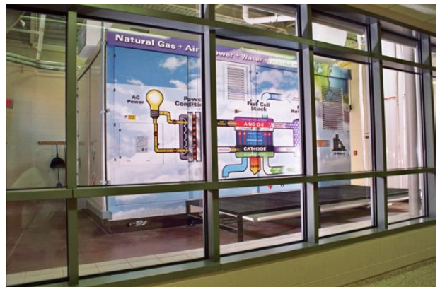
View from School Hallway of the Installed Fuel Cell
