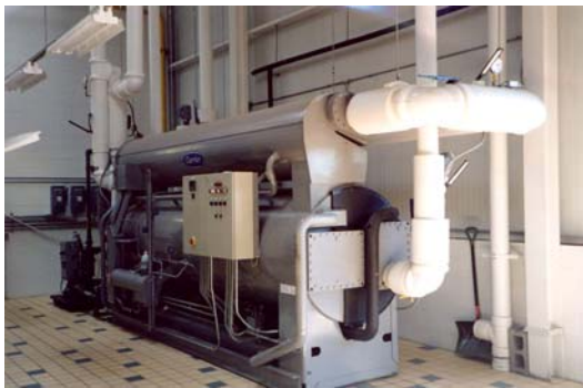
Installed View of Absorption Chiller
