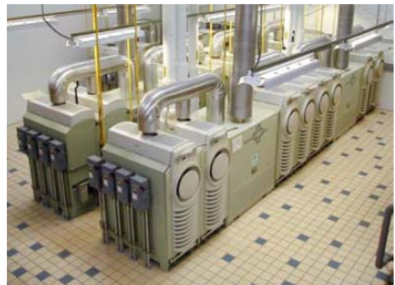
Micro-Turbine Generators and Heat Recovery Modules
