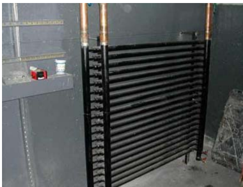
Engine Coolant to DHW Heat Exchanger
