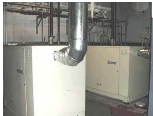
Installed CHP Modules
