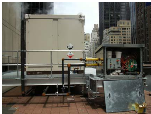
Installed Fuel Cell and Gas Booster
