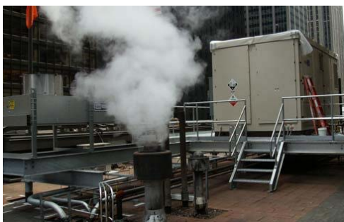
Installed Fuel Cell and Dry Cooler on Left
