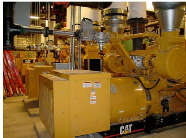
Landfill Gas Fueled Engine-Generator Sets
