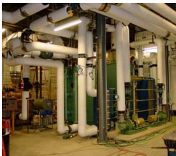
Heat Recovery Components
