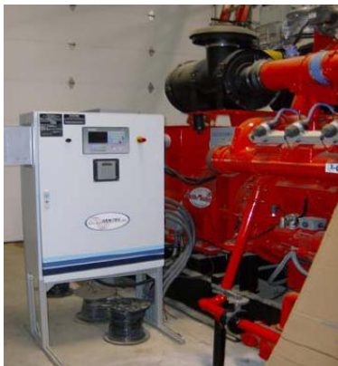
Engine and control panel
