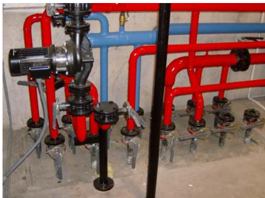
Digester heat piping
