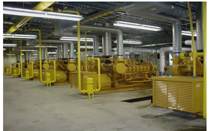
Landfill Gas Fueled Engine-Generator Sets
