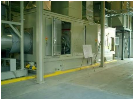
Typical package gas turbine installation
