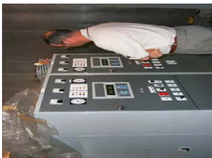
Engine Control Panels
