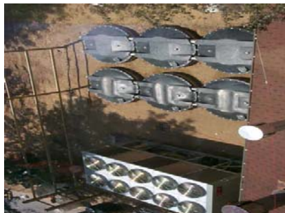
Ice Storage Tanks
