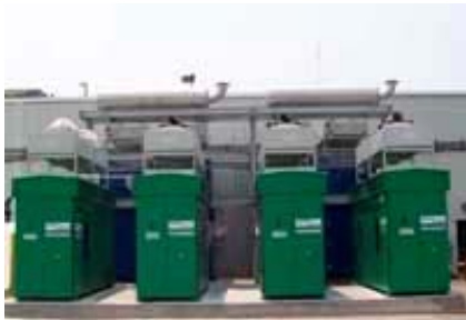
Installed Generator Modules
