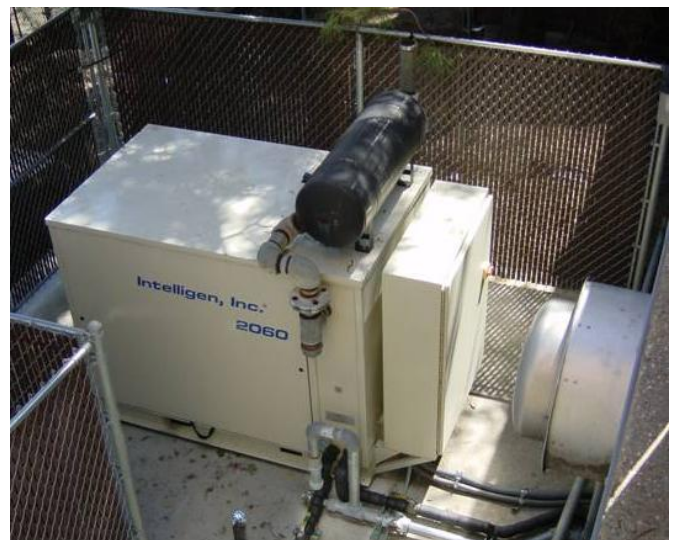
Outside Installation of a 60 kW CHP Module
