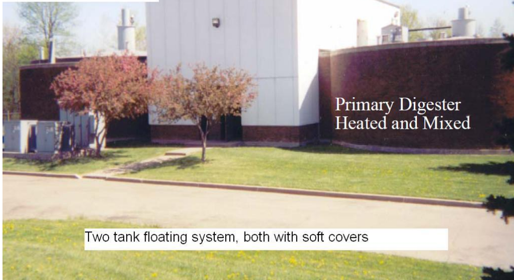
Secondary Digester Gas Storage Cover
